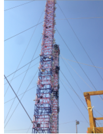
Figure 7 - None of 3 men has fall-out prevention
